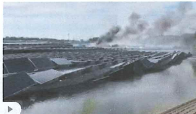
Floating solar power farm catches fire ... abcnews.go.com
