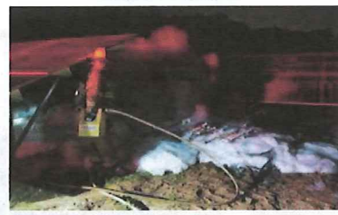
Solar Panel Farm Fire Off ... tacomafire.org
