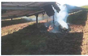
Solar Farm Fire at Sandridge Hill ... pv-stop.com
