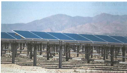
A commercial solar project in San Bernardino County's Lucerne Valley. (Allen J. Schaben / Los Angeles Times)
