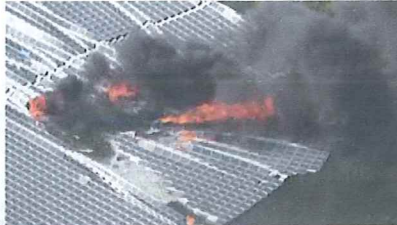
floating PV plant catches fire ... pv-magazine.com
